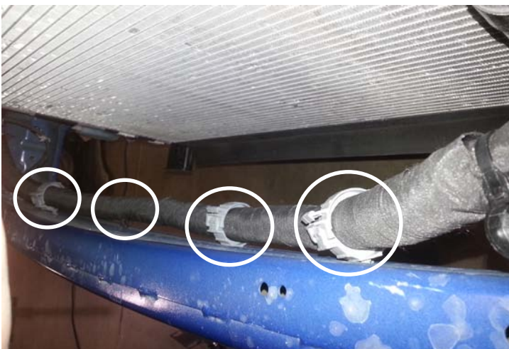
Wiring Harness Retainers
