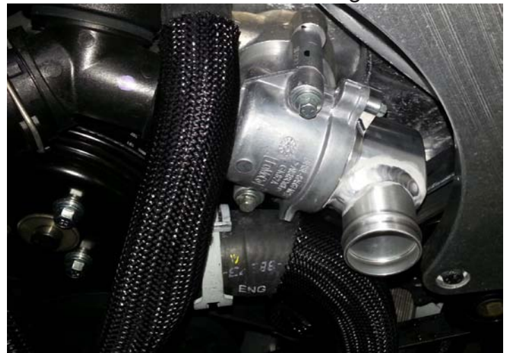
New Thermostat Housing Neck Installed
